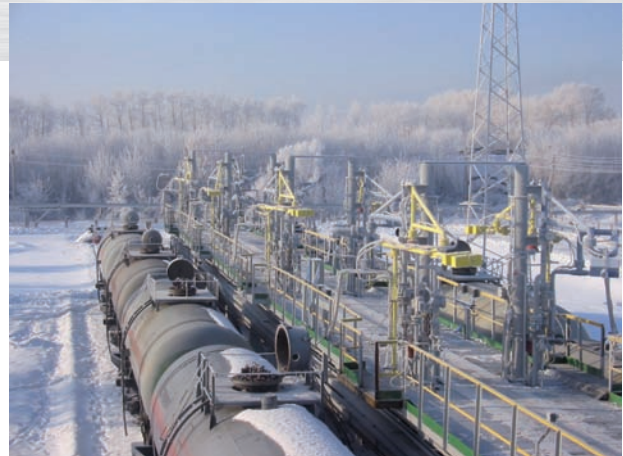
One of the IB Großmann planned and installed railway tanker loading stations.
